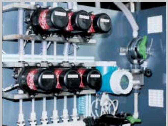
chemical production plant for photographic industry
